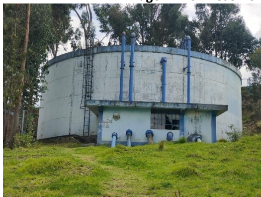
Reservorio Azapampa 2,000 m 3
